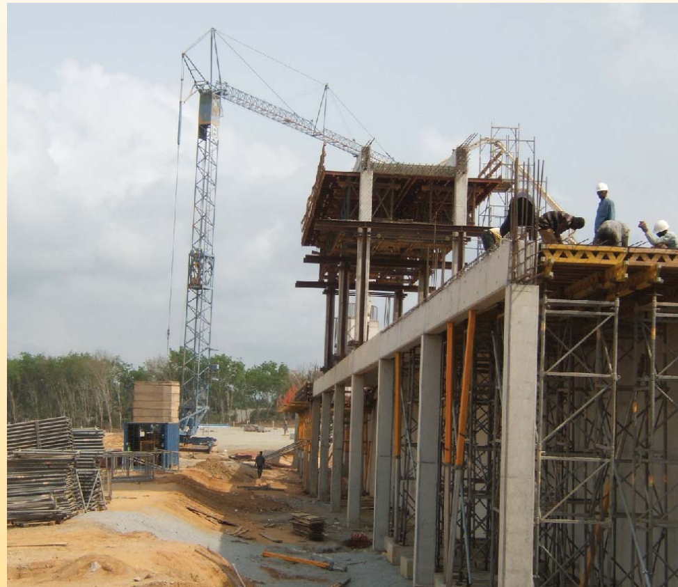
Construction on the Free Trade Zone is well advanced and is scheduled to meet the November deadline.
